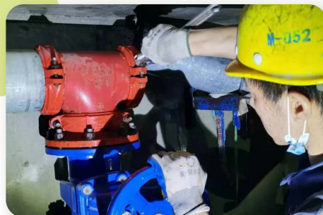
Comprehensive inspection of all equipment operating conditions 全面巡檢各項設備運行狀況
